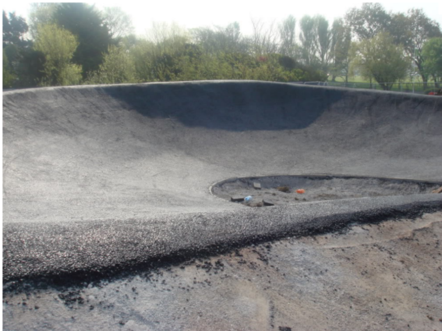
Figure 2: Photograph showing berms tarmac coated. This increases the level of grip on the corners and ensures fewer crashes while turning.
